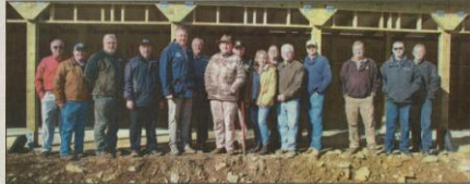
Local leaders met with University System of Georgia Chancellor Dr. Sonny Perdue for a tour of the under-construction Union County Shooting Range last month, pictured here at one of the shooting sheds on the property. Photo by Shawn Jarrard
